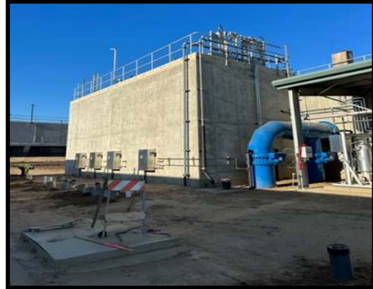
Figure 2: Ozone System – Line Injection Pipework – Access Hatch for Lime
