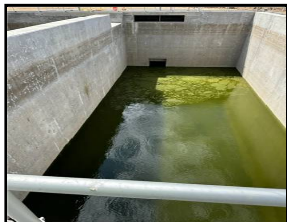
Figure 6: EQ Basin – Dewatered Plant to Begin Disinfection
